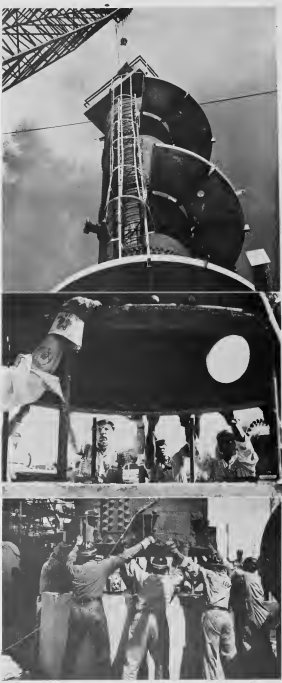
A FIFTY-TON tower over eight anchor bolts. The descent of the tower, which is T-9 at NPFR, must be perfect to align each bolt in the base ring of the tower with each bolt in the foundation. POCO-POCO E ta bal, cu e mas facilidad cu lo por worde spera mientras tratando di laga un tower di cincuenta y cinco ton haba ariba ocho boln pa wante. E bahamento di e tower, cual ta tower T-9 na NPFR, mester ta perfecto pa pone cada buraco den e renchi na base di e tower den tin luga cu cada boln den e fundoshi.
